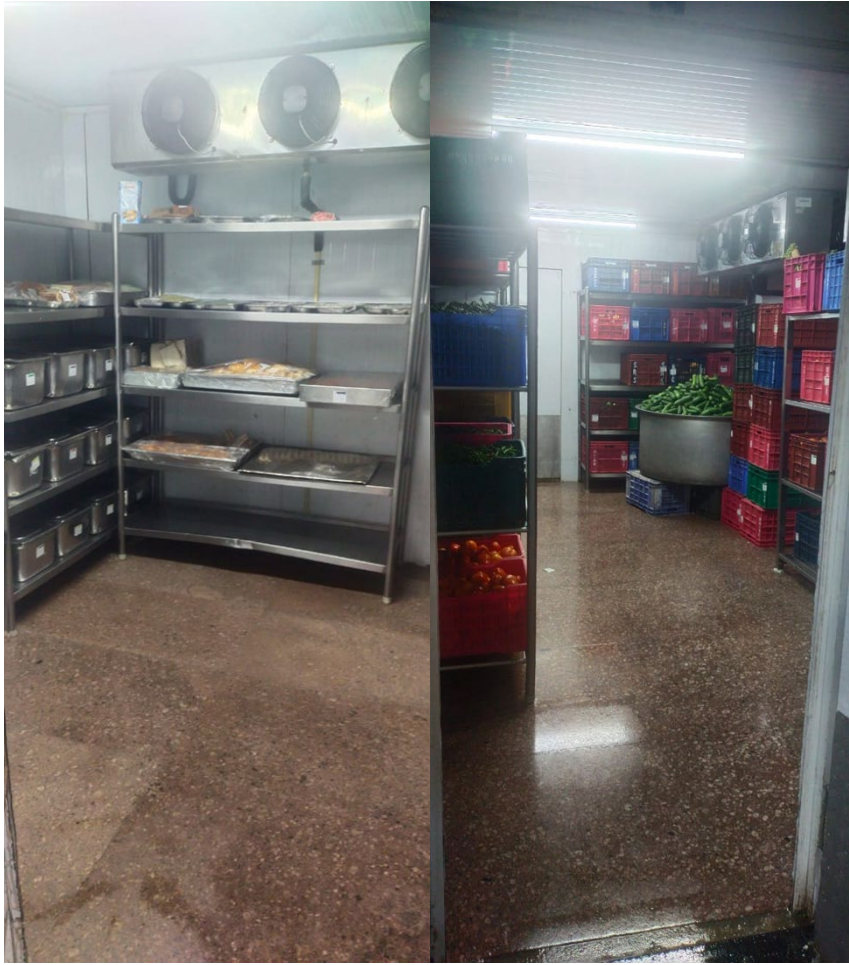
Picture 1: Cold Room for food storage
